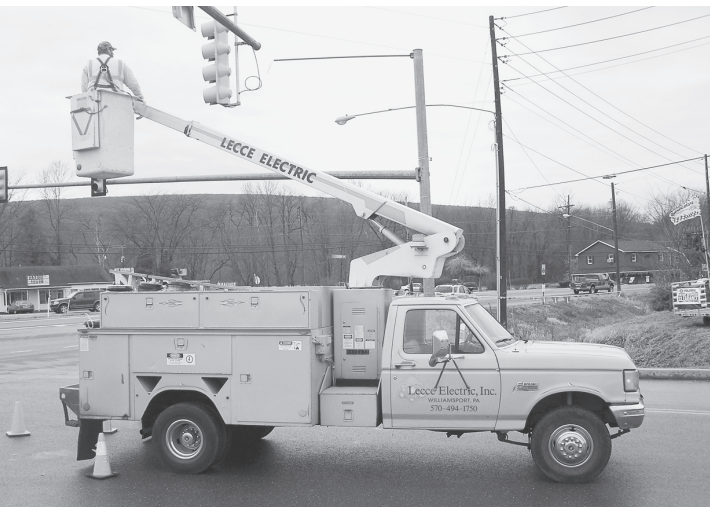
Workers install new LED traffic signal lenses at a major intersection near the Lycoming Mall in Muncy Township, Lycoming County.
